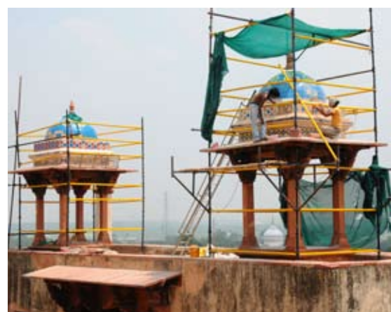
Conservation works at Humayun's Tomb, such as repairing the sandstone platform (top), replacing 20 th century cement flooring with original stone paving (centre) and restoring glazed tiles to the canopies (bottom) are carried out by craftsmen using traditional tools, materials and building techniques.
