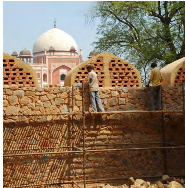
Stone carvers (top), plasterers (central) and masons (bottom picture) used traditional materials building techniques and tools to restore the intention of the Mughal builders
