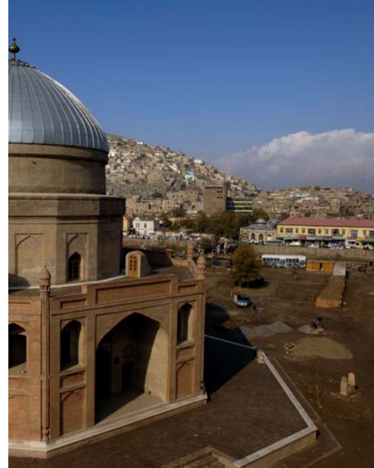
Planting and paving are currently under way in the reclaimed park around the newly-restored mausoleum of Timur Shah in central Kabul
