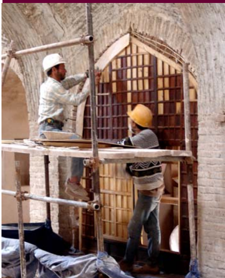
Restoration of damaged oros/ screens on the first floor of the interior space has provided an opportunity to train carpenters
