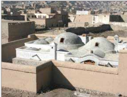
Work on the restoration of the structure of the hammam is now nearing completion
